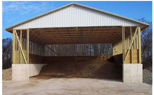
A covered manure storage eliminates runoff.
