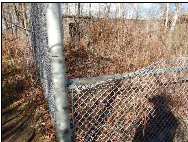
Photo 44 – Exterior Fencing Deficiency (Possible Evidence of Fence Climbing)
