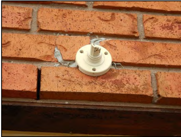
Photo 33 – Broken Security Camera
