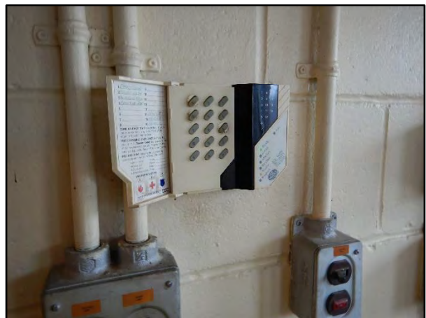
Photo 32 – Security System Keypad Inside Control Building
