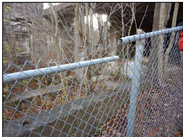
Photo 45 – Exterior Fencing Deficiency
