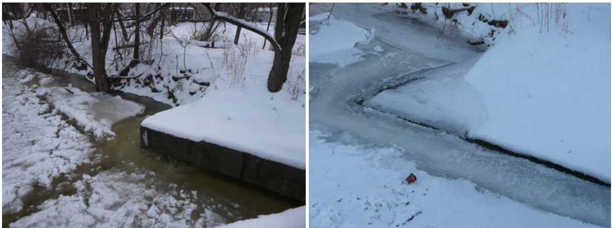
Figure 2-6: Downstream Side of the South Abutment of Thorpe St. Bridge (Left: Jan. 14, 2009; Right: Jan. 16, 2009)
