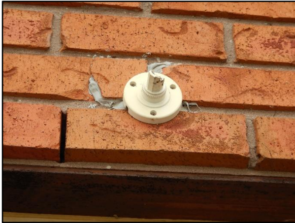
Photo 33 – Broken Security Camera
