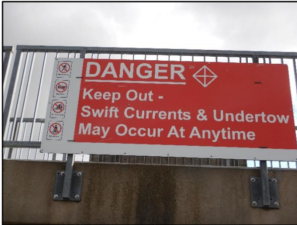
Photo 21 – Public Safety Sign Above Drop Inlet Structure
