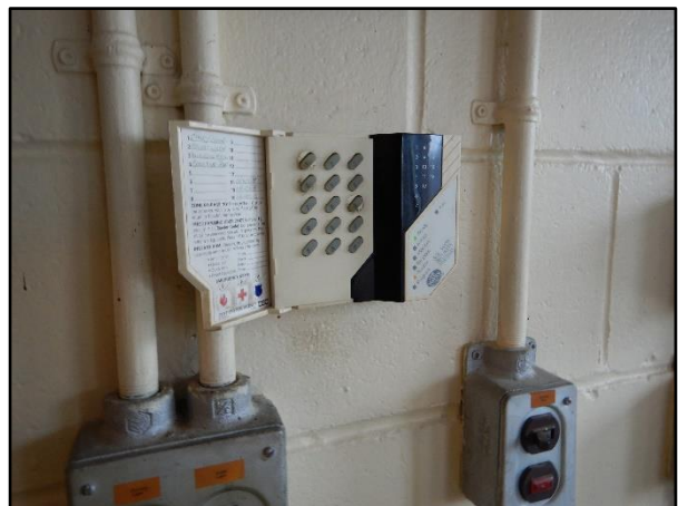
Photo 32 – Security System Keypad Inside Control Building
