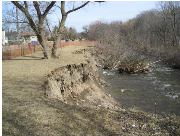
Erosion on Spencer Creek March 12-14, 2010
