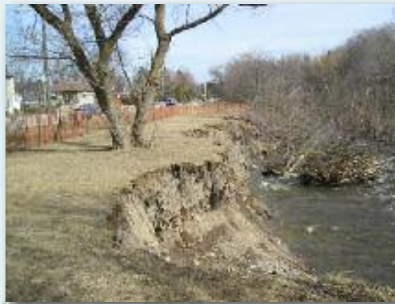
Erosion on Spencer Creek (March 12-14, 2010)
