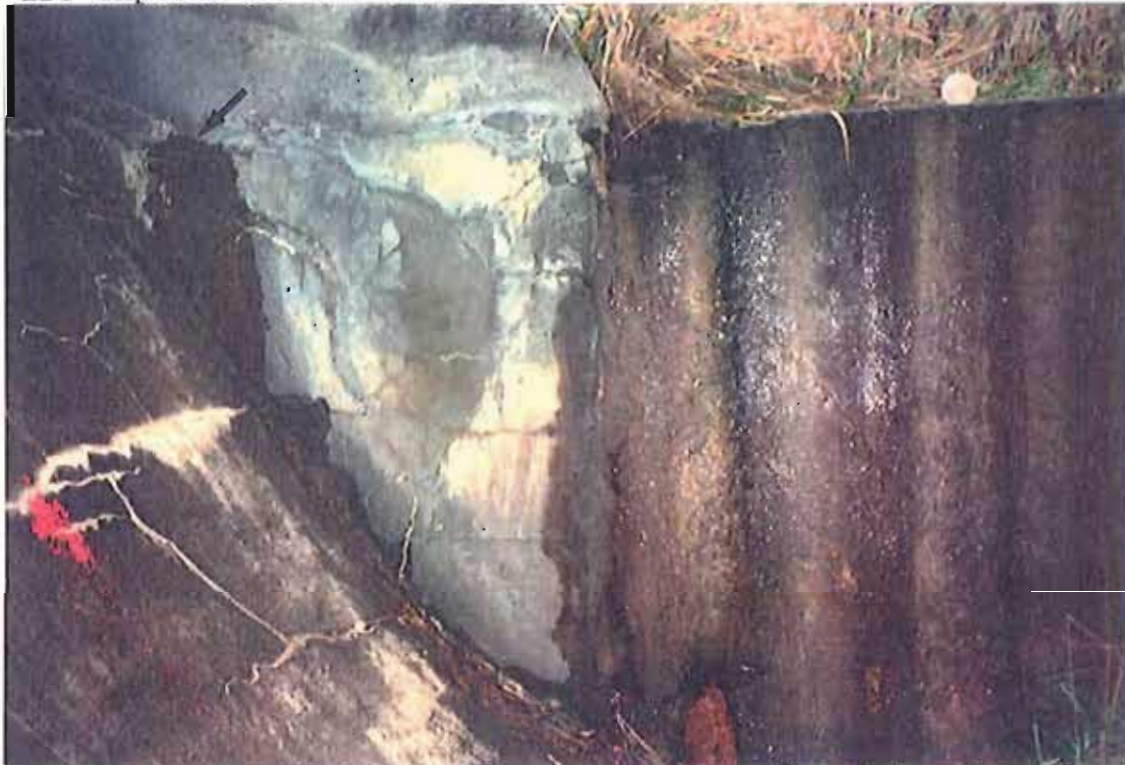
Photograph No. 9 - South face of north abutment and wingwall on the downstream side. Note the water seepage (arrows) through cracks in the abutment. Extensive water seepage also occurs over the face of the wingwall (at right).
