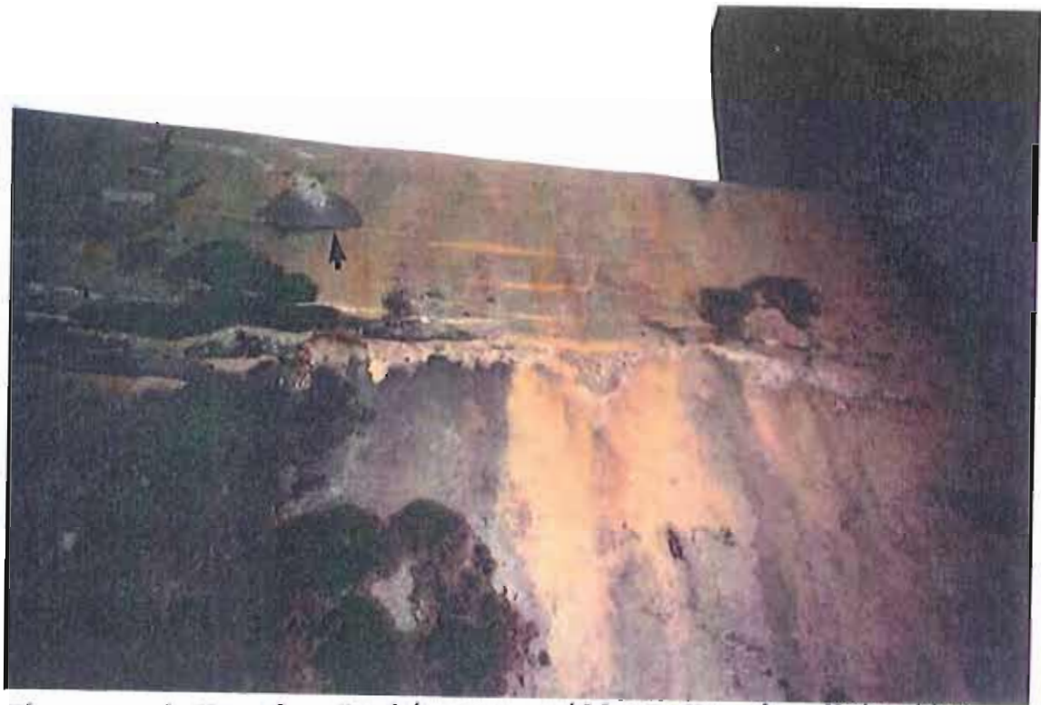
Photograph No. 6 - Looking up spillway No. 4. Note the horizontal and vertical cracking with calcite deposits. Also, the arrows indicate cracks with water seepage.
