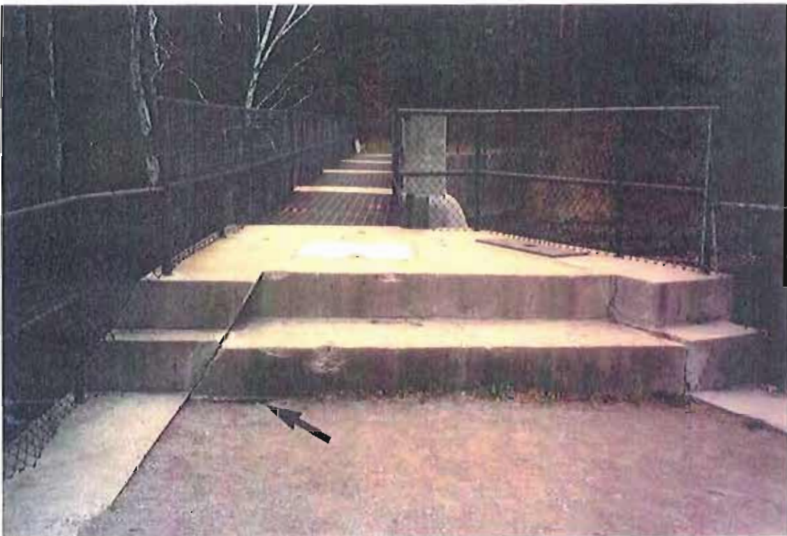
Photograph No.4 - Looking south from the north shore across the walkway over the dam. Note the slight undercutting of the steps at the lower left (arrow).
