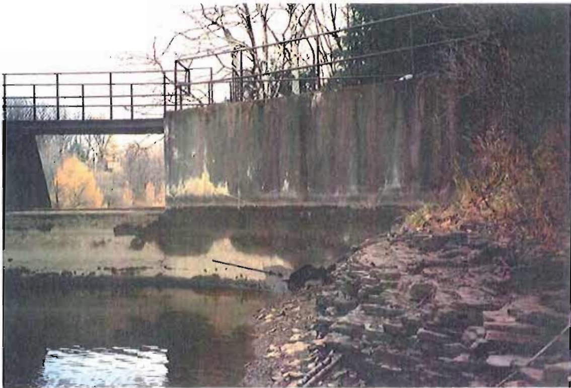
Photograph No.3 - Upstream face of South Abutment at right and spillway No. 4 at left. Note that the intensity of cracking and leaching is less on this face than on the North Abutment. The arrow indicates the location of core No. 4.
