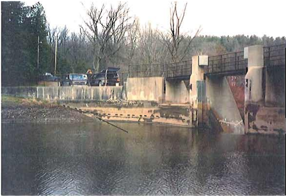
Photograph No. 1 - Upstream face of North Abutment and wing wall show extensive horizontal and vertical cracking with white \text{CaCO}_3 deposits along the length. Core No. 3 (arrow) was extracted below the level of shotcrete repairs (dashed line). Note the epoxy injection into buttress 1 as seen through spillway No. 2.
