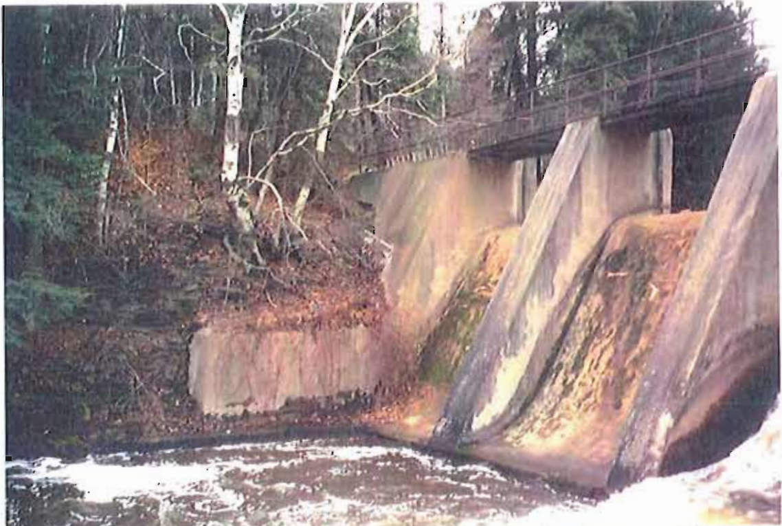
Photograph No. 5 - Downstream face. South shore. Note the cracking and leaching of the south abutment as well as spillway 4 and 3 (fore ground).
