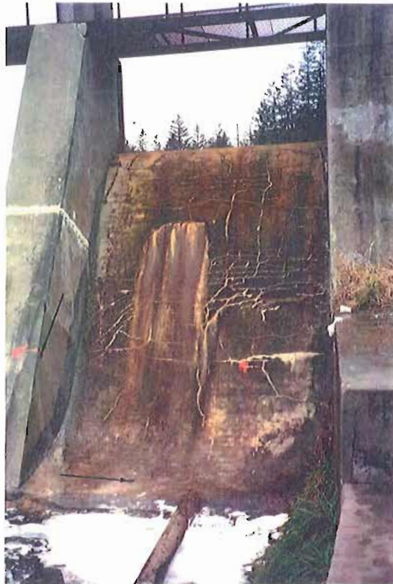
Photograph No. 7 - Downstream face of spillway No. 1. The arrows show the locations of core No. 1 in the buttress and core No. 2 in the toe of the spillway. Core No. 8 was drilled vertically into the top of the buttress. Note the intensity of cracking on the spillway face as the result of freeze-thaw and wetting-drying effects.
